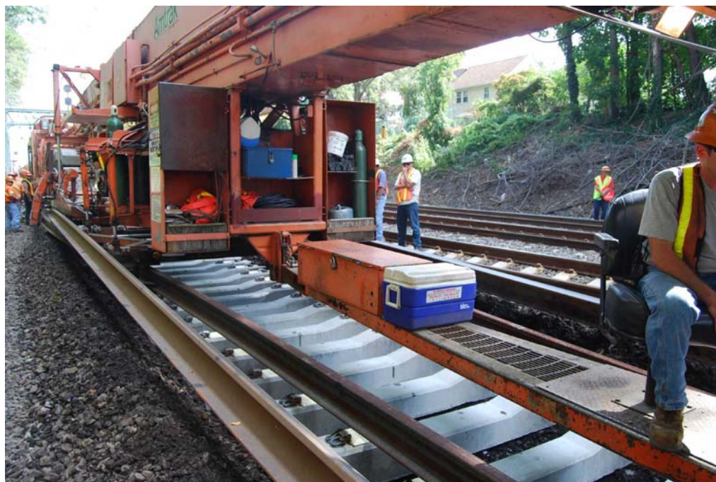
Amtrak 30 Year Old Track Relaying Train at work near Bryn Mawr, west of Philadelphia (Note this was a weekday operation with all adjoining lines open to traffic and OLE live)
