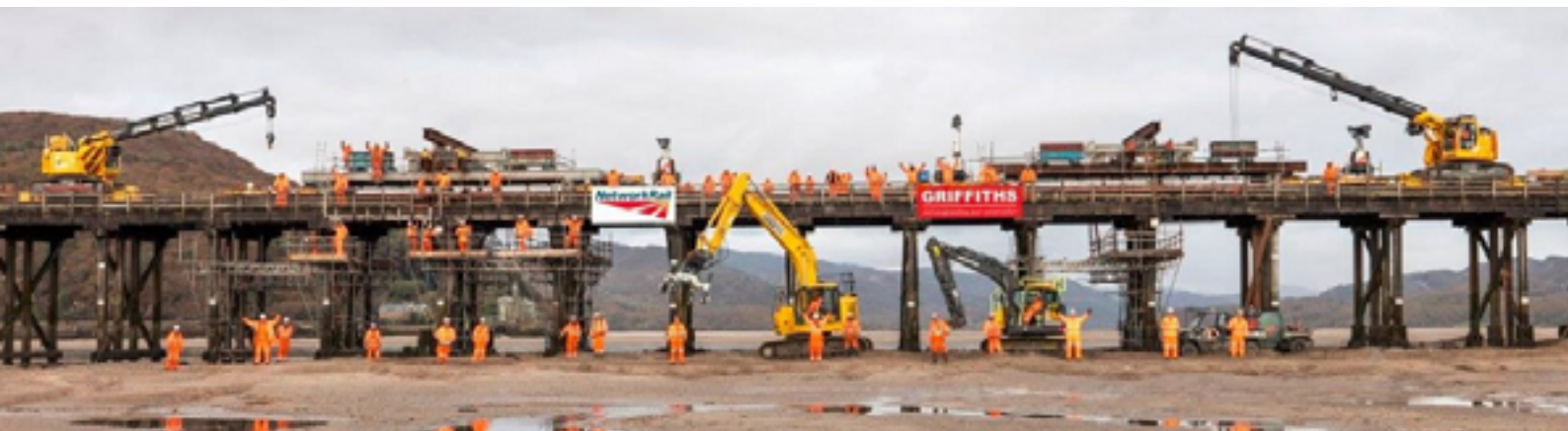
Work on Stage 1 of the Barmouth viaduct in late 2020, was undertaken with pandemic restrictions in place
