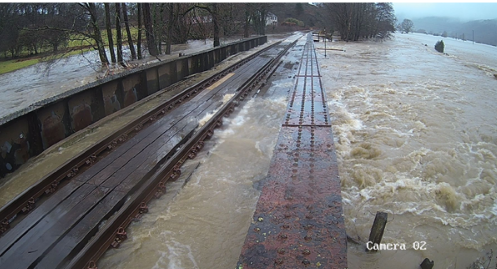
Camera footage of the Black Bridge in January 2021 shows flood water over the rail line
