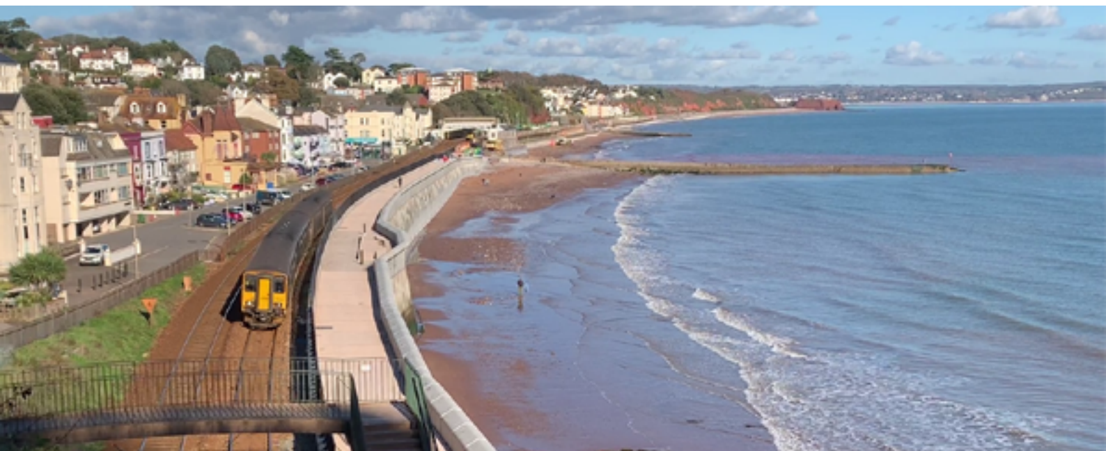
The completed first phase of the 360 metre section of the Dawlish sea wall in early July 2020
