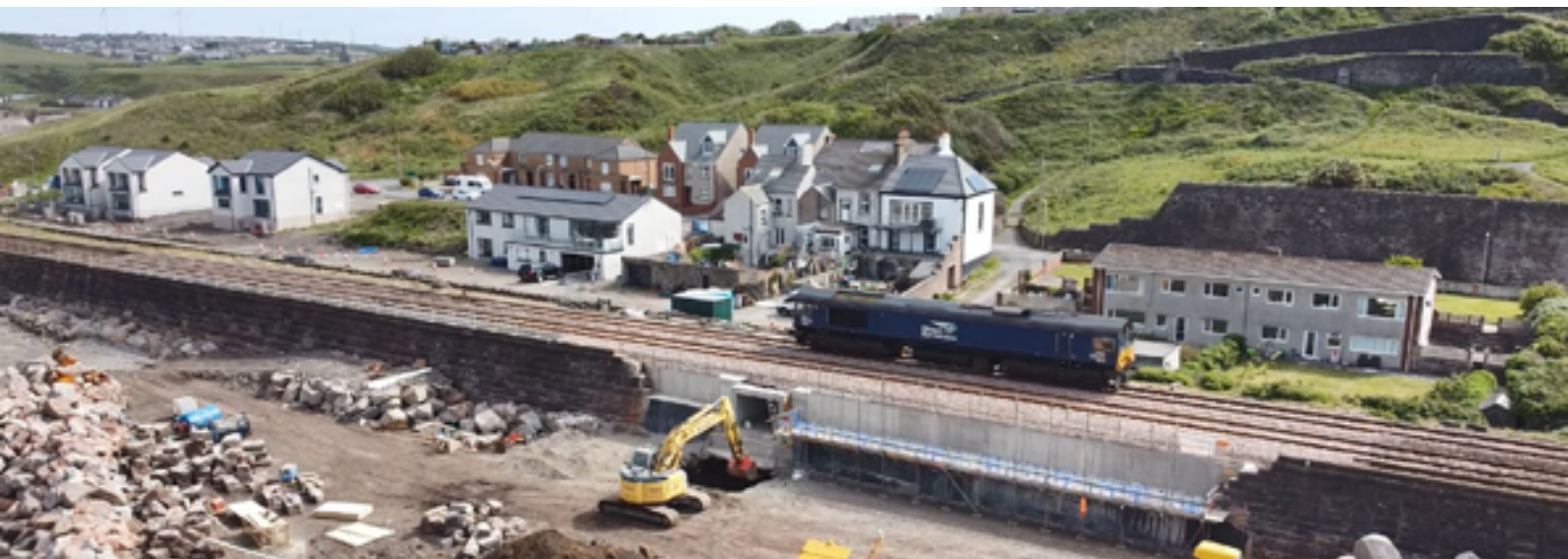
Work on a railway bridge at Parton on the Cumbrian Coast Line following storm damage in early 2021.
