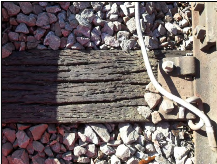
Figure 5-4 Decayed and splitting timber bearers
