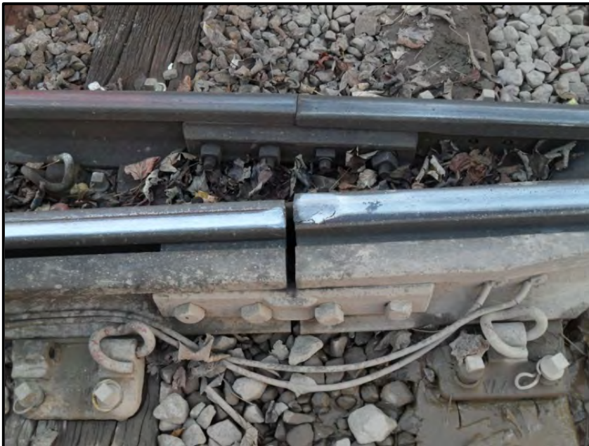
Figure 5-16 Rail head spalling at crossing joint
