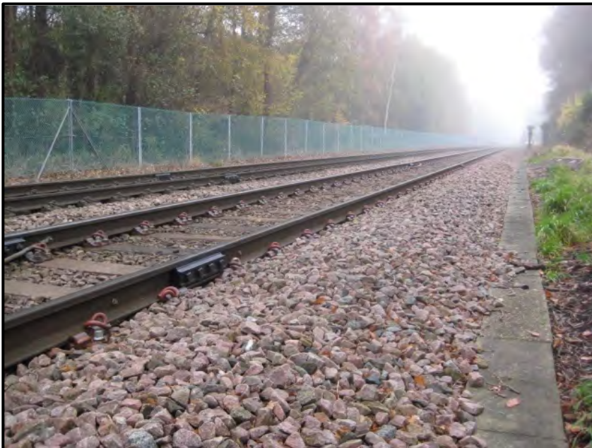
Figure 5-27 The line to be refurbished nearest to the camera. (Note new fastenings.)
