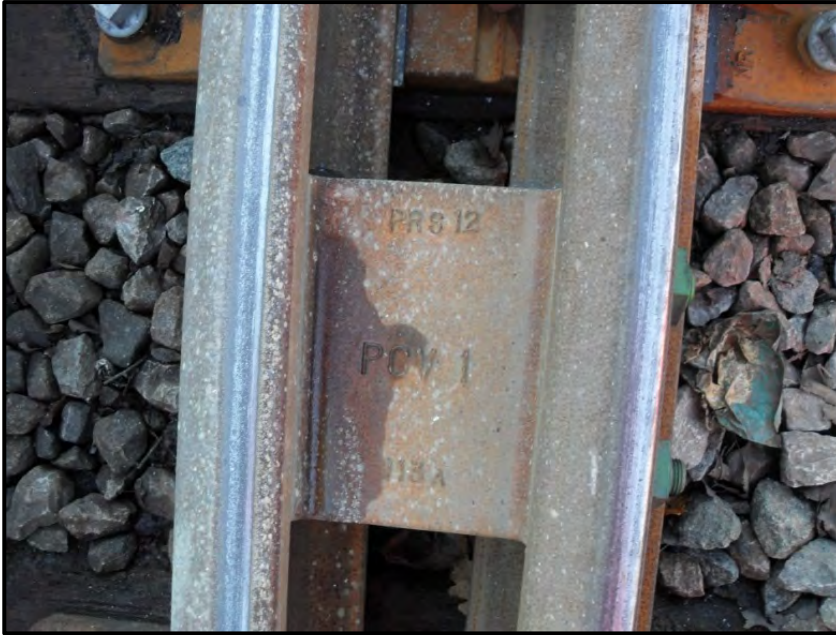
Figure 5-3 2012 Switches with strengthen blocks
