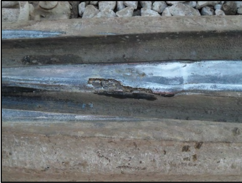
Figure 5-17 Degraded weld repair to crossing nose
