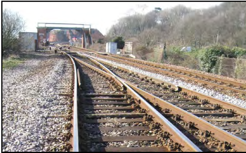
Fig 5-30 S&C at the Plymouth end of Dawlish Warren Station (Down Loop) 921 points and 922 crossover
