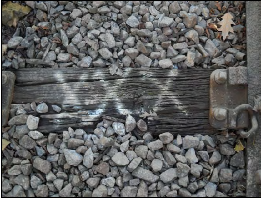
Figure 5-13 Typical Split and Decayed Timber
