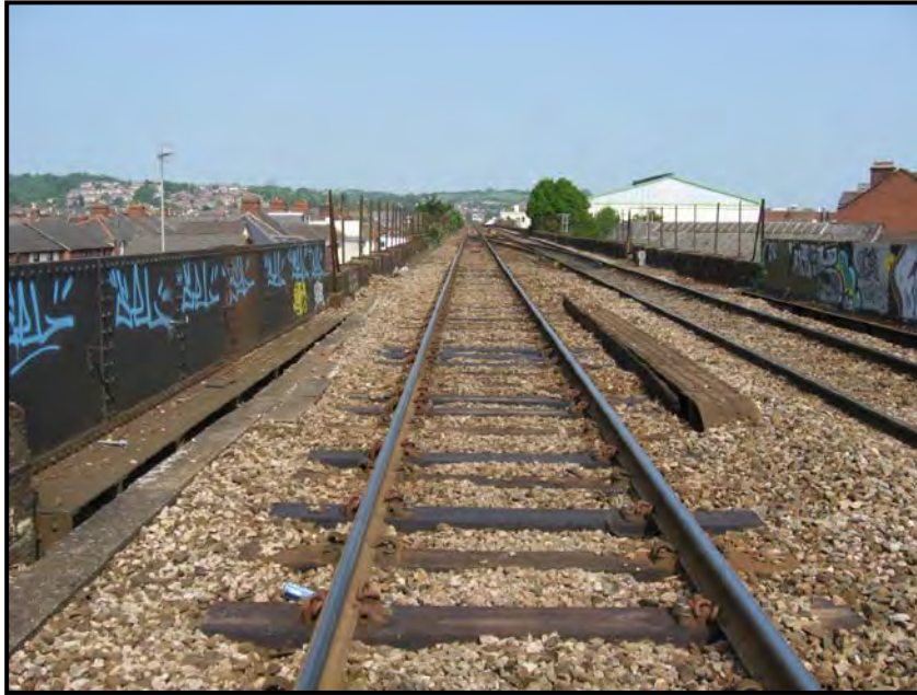
Fig 5-28 Exeter St Thomas. Note that some sleepers have already been changed.
