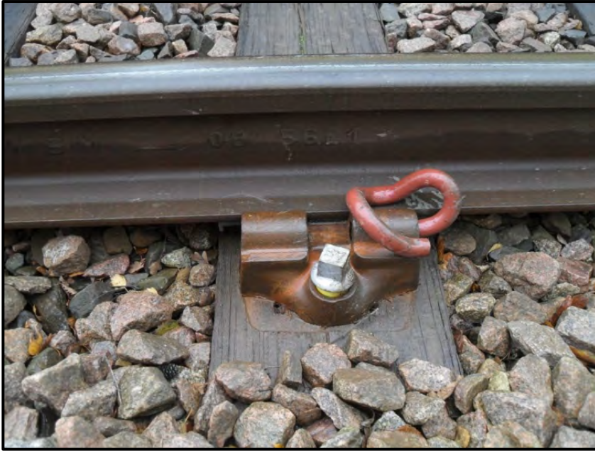
Figure 5-26 Pan 11 baseplate replacement for Pan 8. (Note that the rail is one of two 60ft lengths replaced in 2009.)
