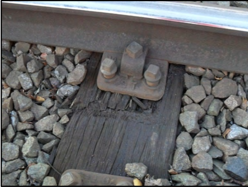
Figure 5-6 Typical poor timber condition in 5A Pts
