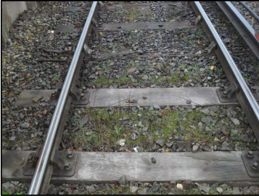
Figure 5-23 Poor ballast conditions: Wet beds and vegetation in 4ft.
