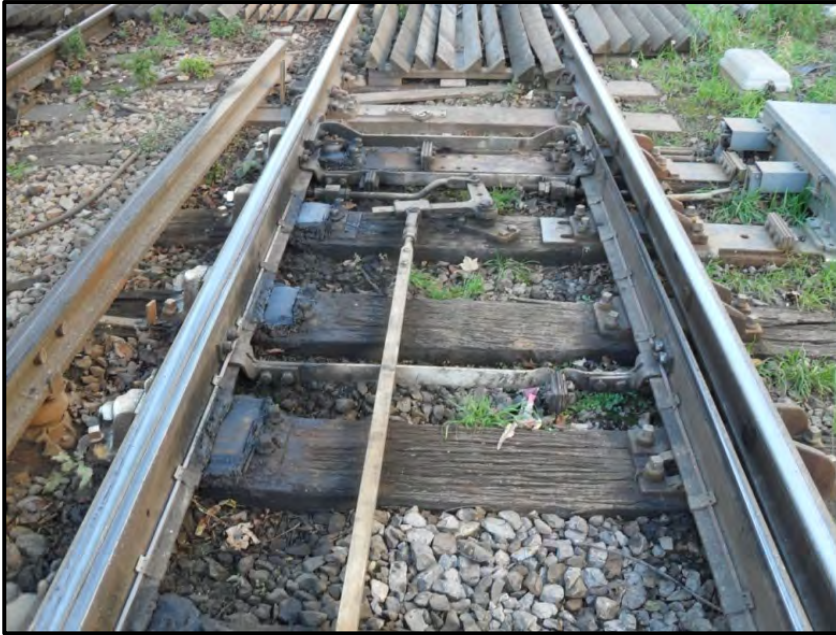
Figure 5-11 637 Pts Left hand switch (RH as viewed) replaced – note differing slide chair blocks.
