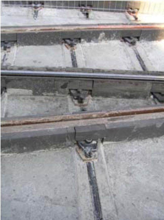
(a) Concrete sleeper fastener adjustment slots
