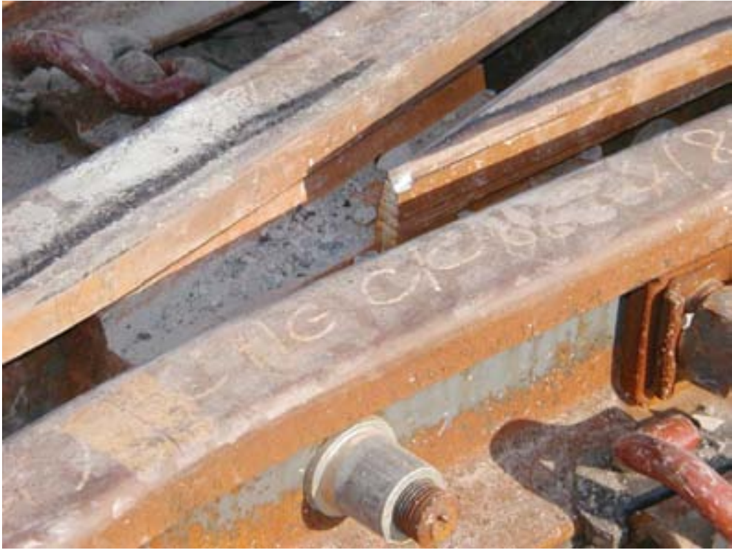
J Brown Figure 8.21 Turnout crossing nose of at Station Street, NET (08.04.03)
