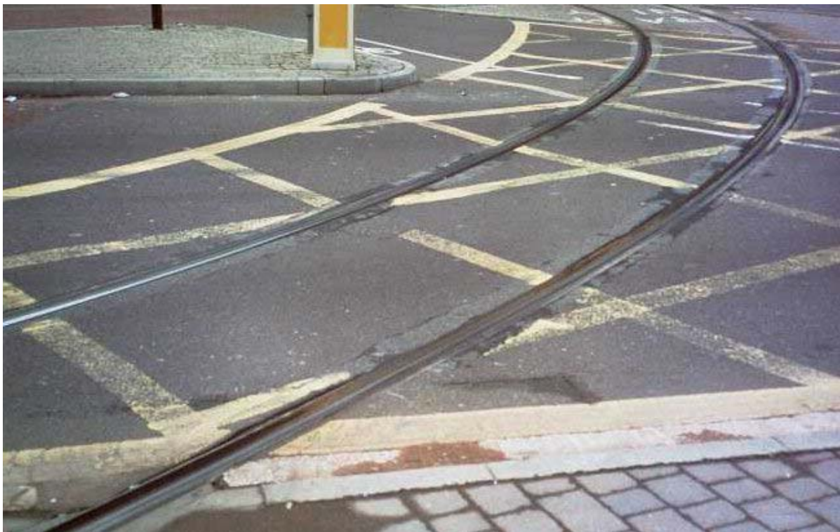
Figure 3.3 Grooved rail track at Croydon, Croydon Tramlink
