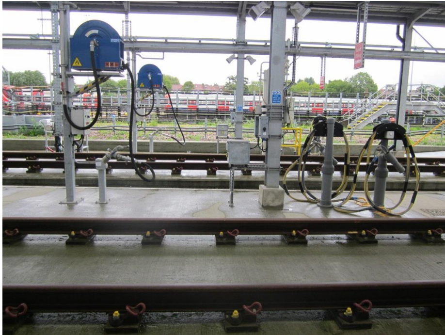
Conductor rail substantially cut back in vicinity of sanding and tanking point
