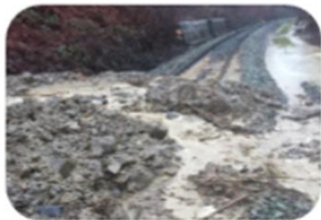
Heavy rain can cause embankment failure and landslides
