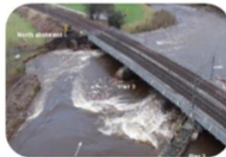
Flooding can cause erosion, destabilising bridges
