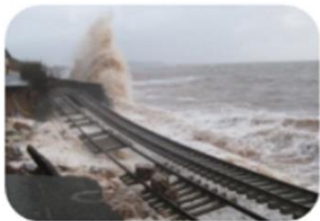
Waves can damage coastal infrastructure
