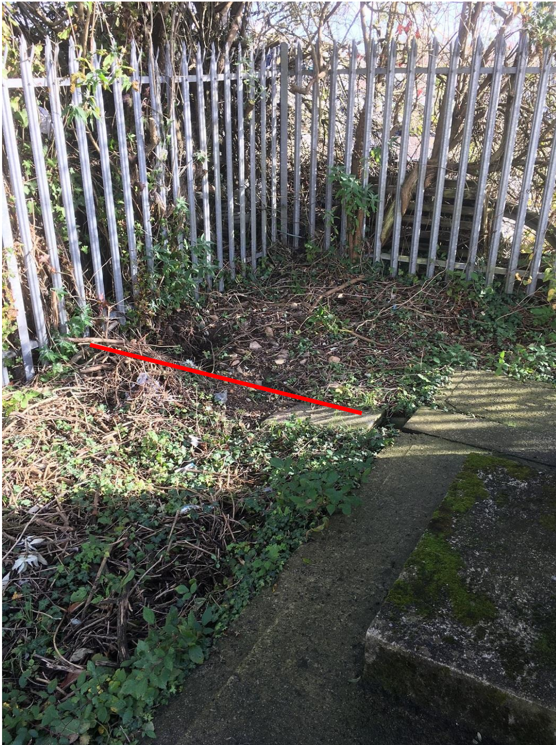
Troughing route. I'm unsure if this continues under the fence as it was overgrown.
